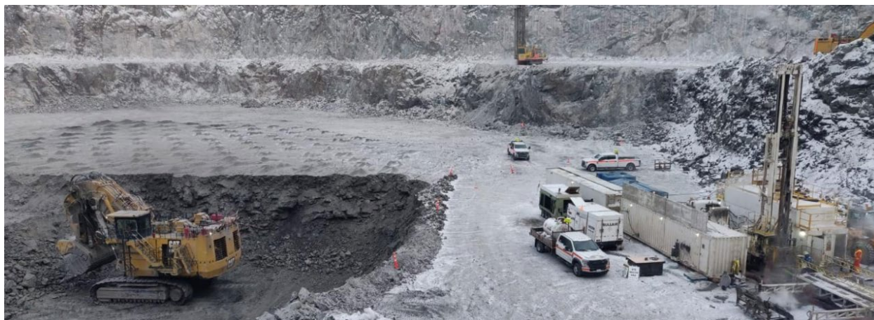
Figure 3 - Sable open pit operation (left) and the completed reverse circulation drilling program (right). A similar set-up will occur next week for the commencement of the delineation and geotechnical Sable underground drill program.
